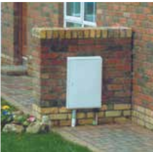
Domestic meter box
