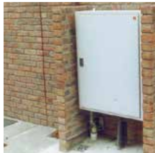
Six meter cabinet
