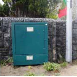
District Regulating Installation (DRI)
